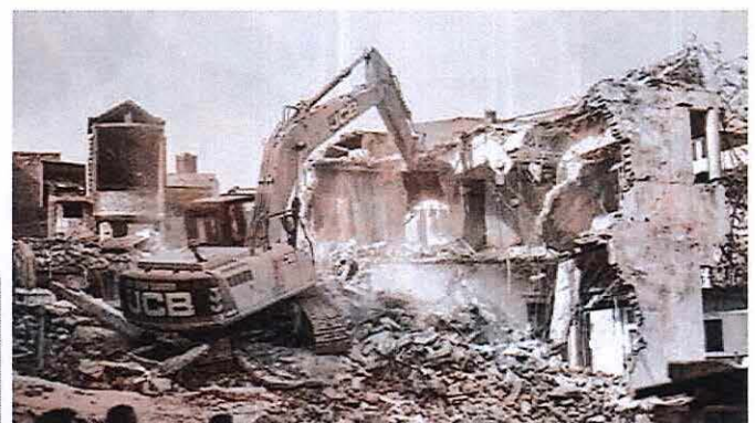
In Prayagraj, the civic body on Sunday demolished 'illegally constructed' residence of Javed Ahmed, a local leader who was allegedly the key conspirator of violent protests against now-suspended BJP leaders
